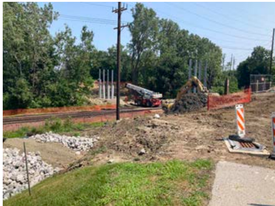
Looking east across to Garrison Hill shows the extent of the excavation for the new bridge to the Veterans' Cemetery.
