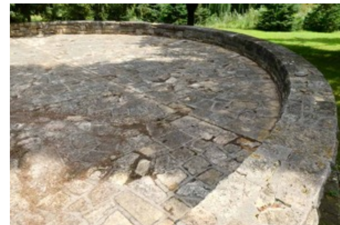
The stonework by the WPA and the CCC at National and state Parks in the 1930s and 40s have withstood the test of time. Garrison Hill can recapture a similar look and level of craftsmanship employed by these agencies.
